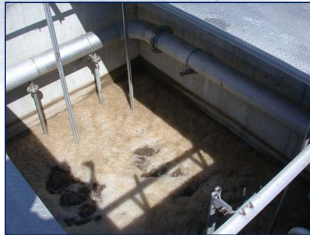
MBR Basin - aerobic zone
