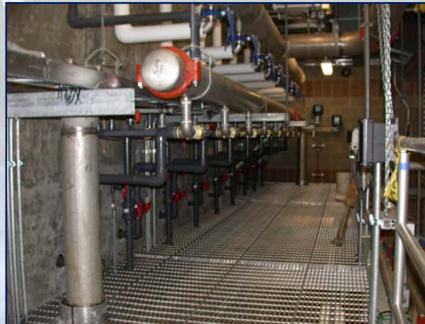
MBR Pipe Gallery - permeate and air piping
